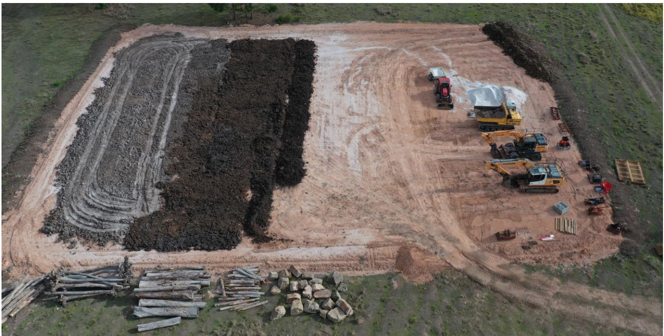
Figure 4. Acid sulphate spoil treatment pad at site 6. Lime application and mixing at 5kg/m 3 spoil.
