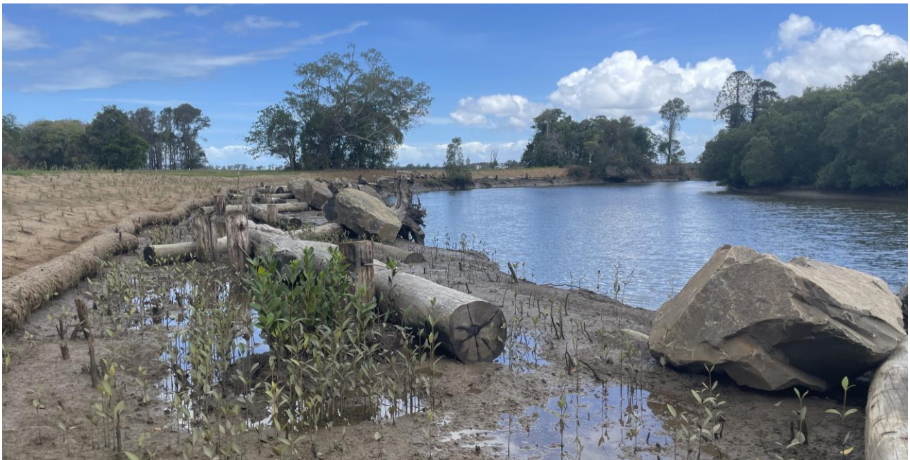
Figure 2. Site B1 after work, November 2023. Dense mangrove saplings in the foreground were translocated within the site during earthworks, while sparse saplings are natural recruits from the Spring 2023 grey mangrove fruiting event.
