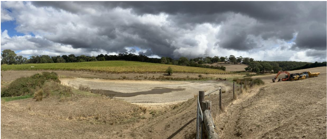
Figure 4 Mobilized heavy machinery, in preparation for a Dam removal in the Bremer River Catchment.
