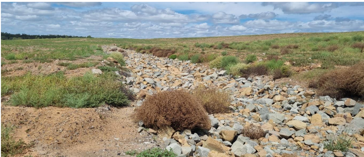
Figure 2: Small chute drain using rock from borrow source after processing (design life – 10 years).
