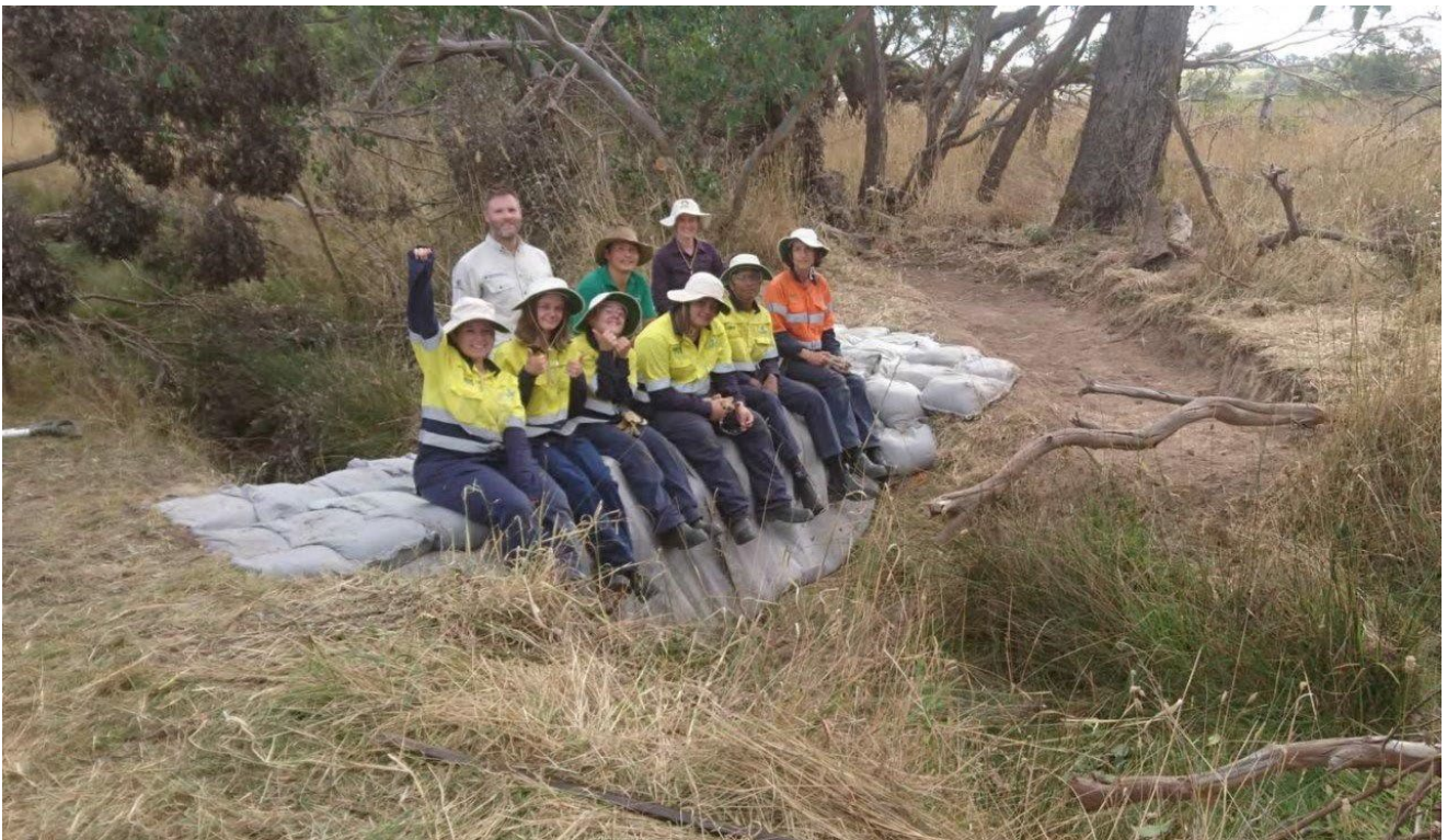
Figure 4. Community volunteers and a recently completed sandbag structure, 5/4/2017. A cutting has been made through the spoil mound of the drain, to the right of the structure, to facilitate lateral flow into the natural creek meanders.
