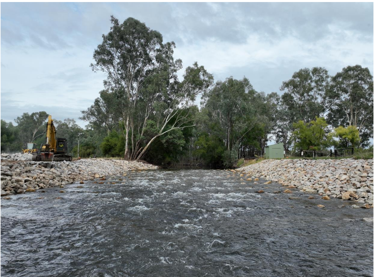
Figure 3. Looking upstream over the fishway
