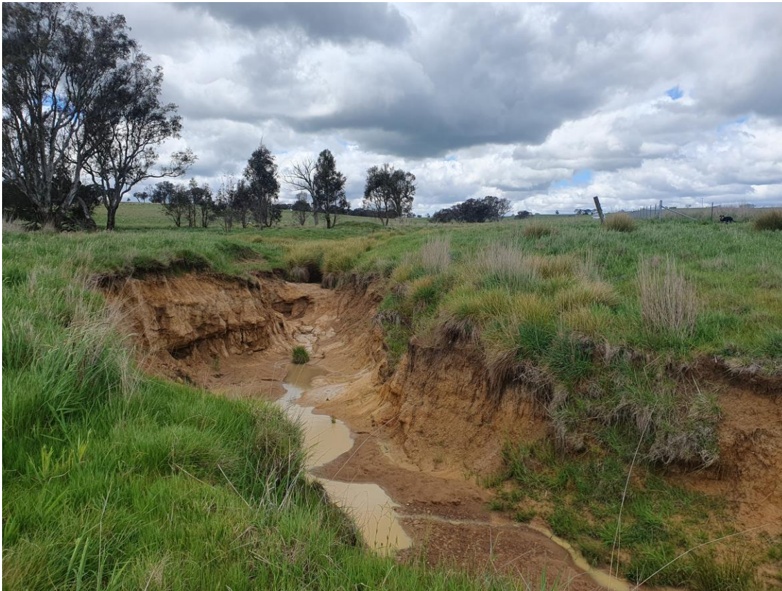
Photo 2 – An example of erosion on Nunick Nunick Creek, which flows into the Boorowa River.
