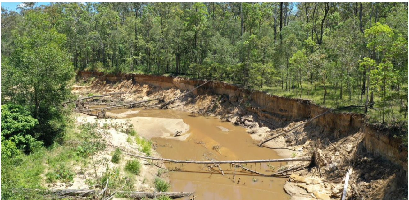
Figure 1. Oxley Creek in the upper erosion zone through the Greenbank Military Training Area
